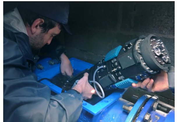
ACWA Robotics employees work with the Pathfinder robot on a water pipe.
