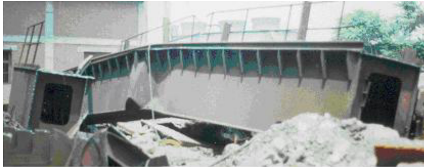
Figure 1. A photo of the auxiliary beam with the deformation
