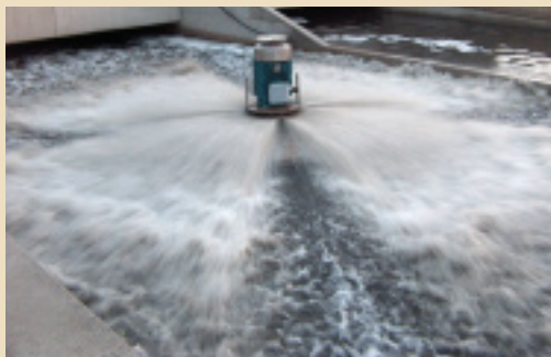
The surface aerator of this bio-reactor is used to resuspend the solids bed from within an aeration lane and to entrain air into the reactor.
