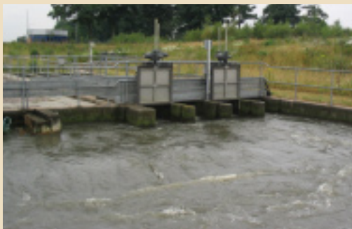
The inlet works for a large ASP illustrates the typical scale.
