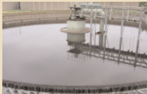
Activated sludge is settled out in this clarifier. Flow enters the tank from the top and flows radially outward.
