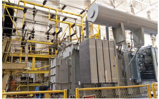
Transformer from Pennsylvania Transformer Technology
