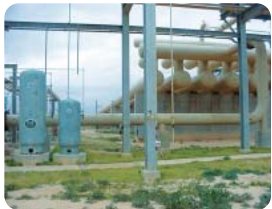
This view of the slug catcher at the BG Hannibal terminal shows the inlet pipe and header as well as the short separation fingers above the much longer liquid fingers.
