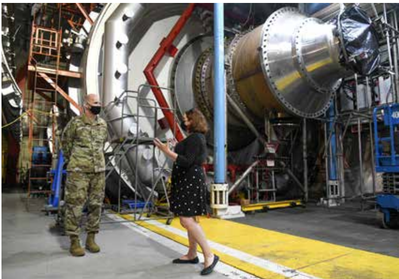
Rachel Garrard, a test manager with the Propulsion Test Branch of Arnold Engineering Development Complex (AEDC), explains how the C-1 altitude engine test cell works to Maj. Gen. Evan Dertien, commander, Air Force Test Center. In C-1, large military and commercial engines are tested at simulated altitude conditions. U.S. Air Force photo by Jill Pickett
