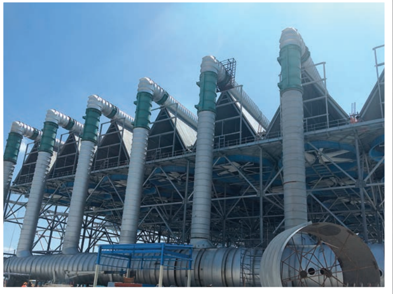
Air-cooled steam condensers
